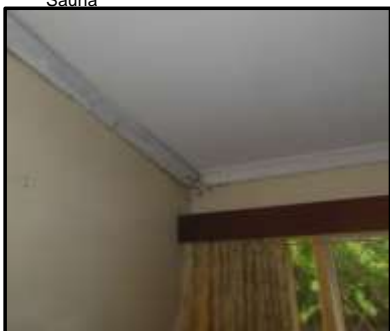
Water leak and damage
