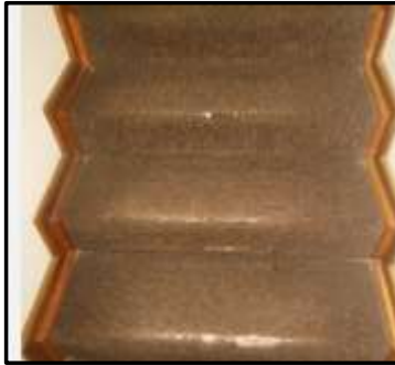
Damage to carpet
