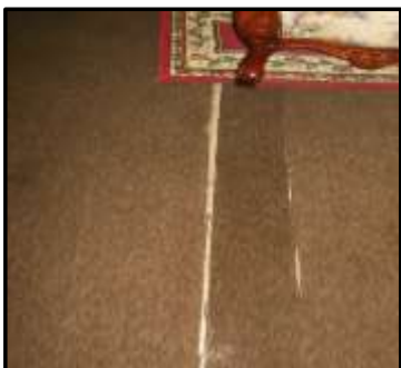
Damage to carpet
